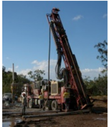
DR 14 getting meters in the Leichardt Ranges. The crew have settled down to the job of drilling
