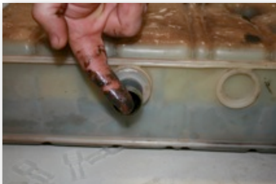
More oily sludge from the Auxiliary Compressor. When you conduct your daily pre-starts, physically check each component to ensure its serviceability.
